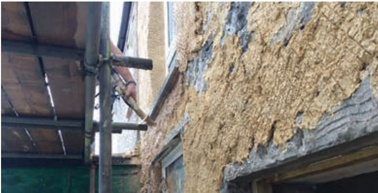
External wall dubbed out by harling prior to pumped application of render ©Peter Draper
